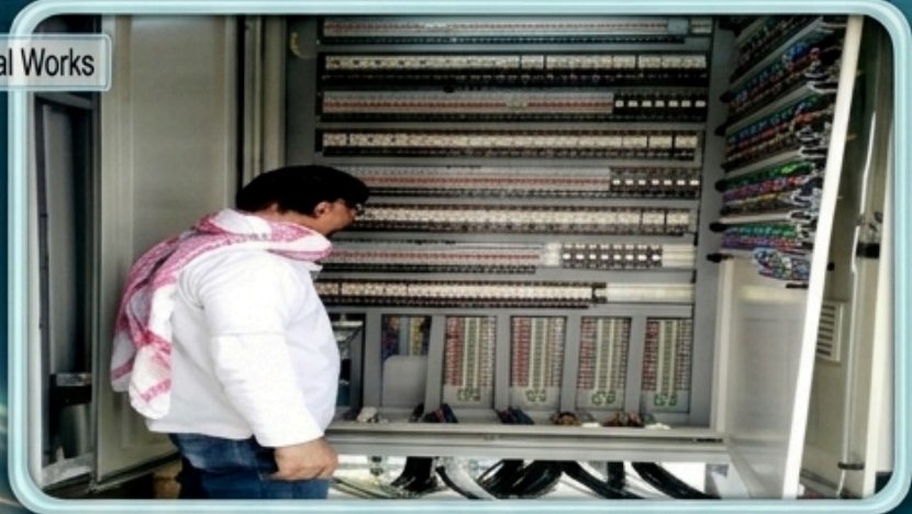
PROJECT NAME - Hotel Electrical Works
